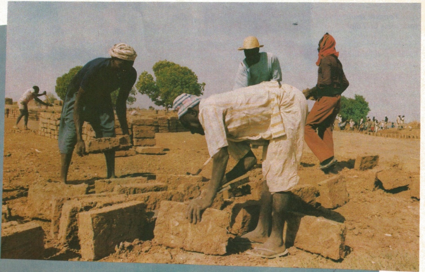
Brick construction under way at Am-Nabak so that the peasants can build irrigation canals. Prior to building the canals they cleared the lots of land given by the government. This project has helped the peasants become self-sufficient in food production.
